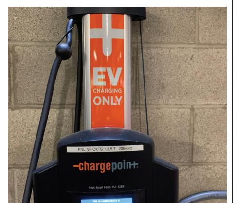
EV charging station in The Alhambra parking garage.
